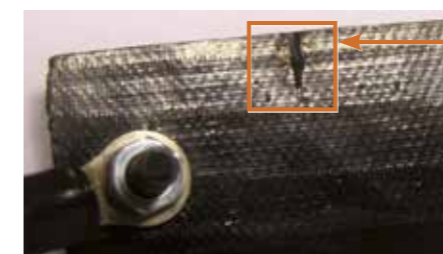
230 VAC Fault with arc fault protection: only cosmetic damages appears
